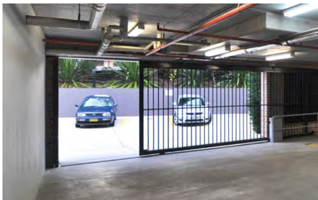
Figure 3J.4 Permeable roller doors allow for natural ventilation and improve the safety of car parking areas by enabling passive surveillance
