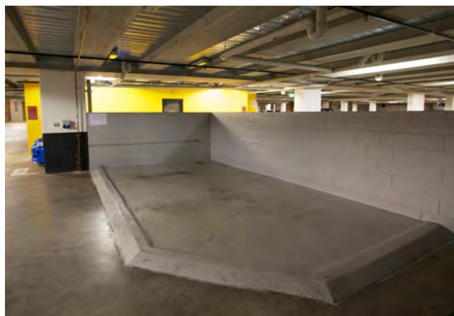
Figure 3J.7 An example of a car wash bay integrated into the basement car park of a residential apartment building
