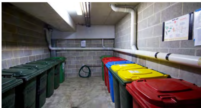
Figure 4W.4 Well designed, easily accessible and clean waste and recycling rooms improve the collection and management of household waste
