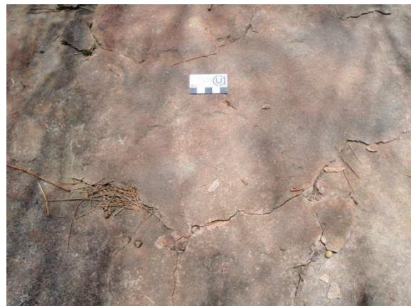
Plate 40. View north, showing eastern circular engraving and exfoliation on the south-western edge
