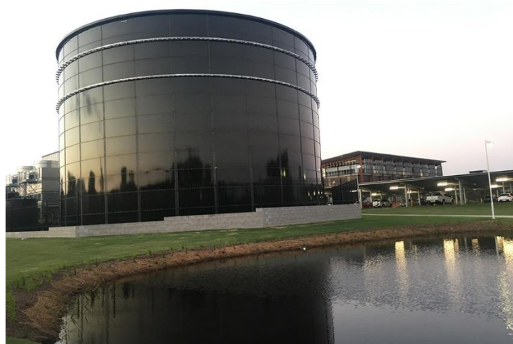
Figure 33: Chilled Water Storage Tank - University of the Sunshine Coast
