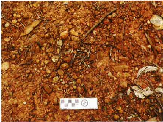
Figure 5.179 Compacted clay and gravel surface, exposed in unused area of road reserve, on the east side the Canal.
