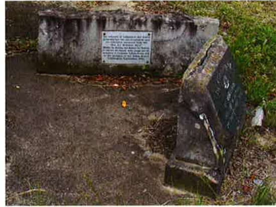
Figure 5.80 The sandstone base of the memorial is suffering significant deterioration, including contour scaling.
