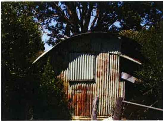
Figure 5.172 Nissen hut on Bringelly Road; view of the west elevation with original cladding and windows.
