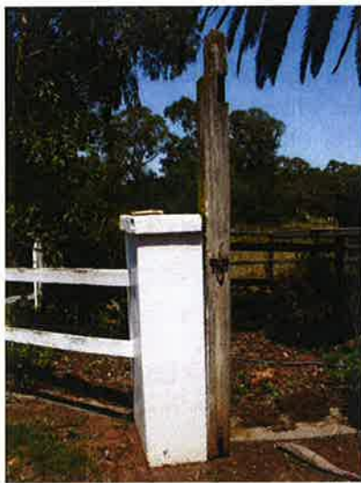
Figure 5.153 Remnants of timber gate post.
