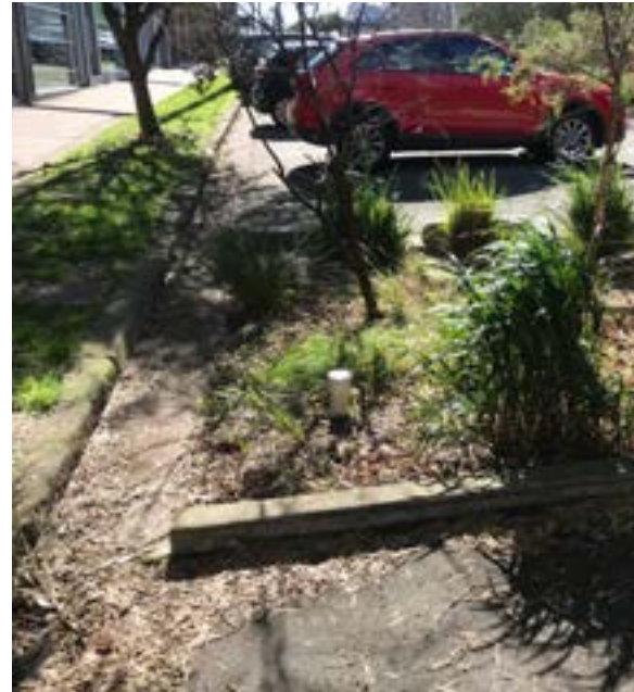
Figure 47: Kerb side opening allows stormwater to enter soil
