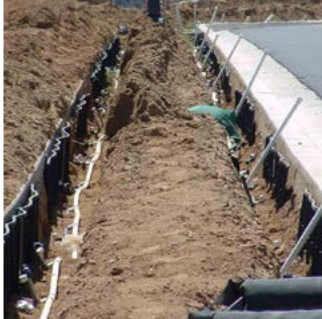
Figure 56: 'Root Barrier on Brown Road: Petaluma, California 2013' by DeepRoot Green Infrastructure
