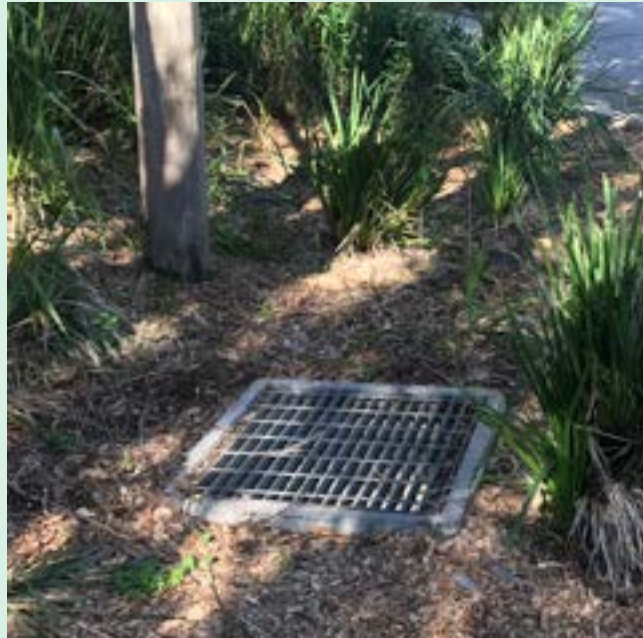
Figure 50: Excess water exits via overflow outlet
