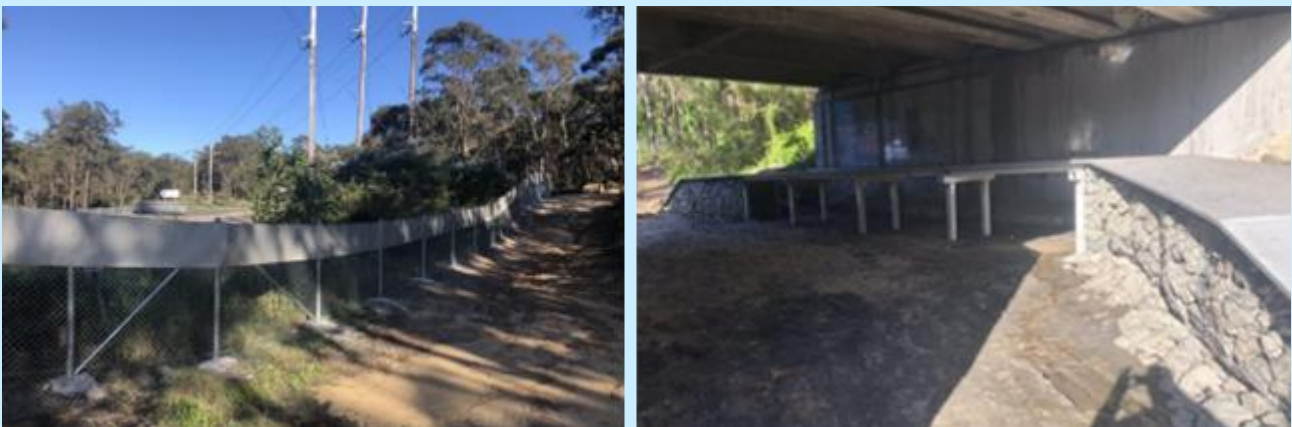
Figure 9. New fencing (left) and a new koala underpass (right) at Kings Falls Bridge
