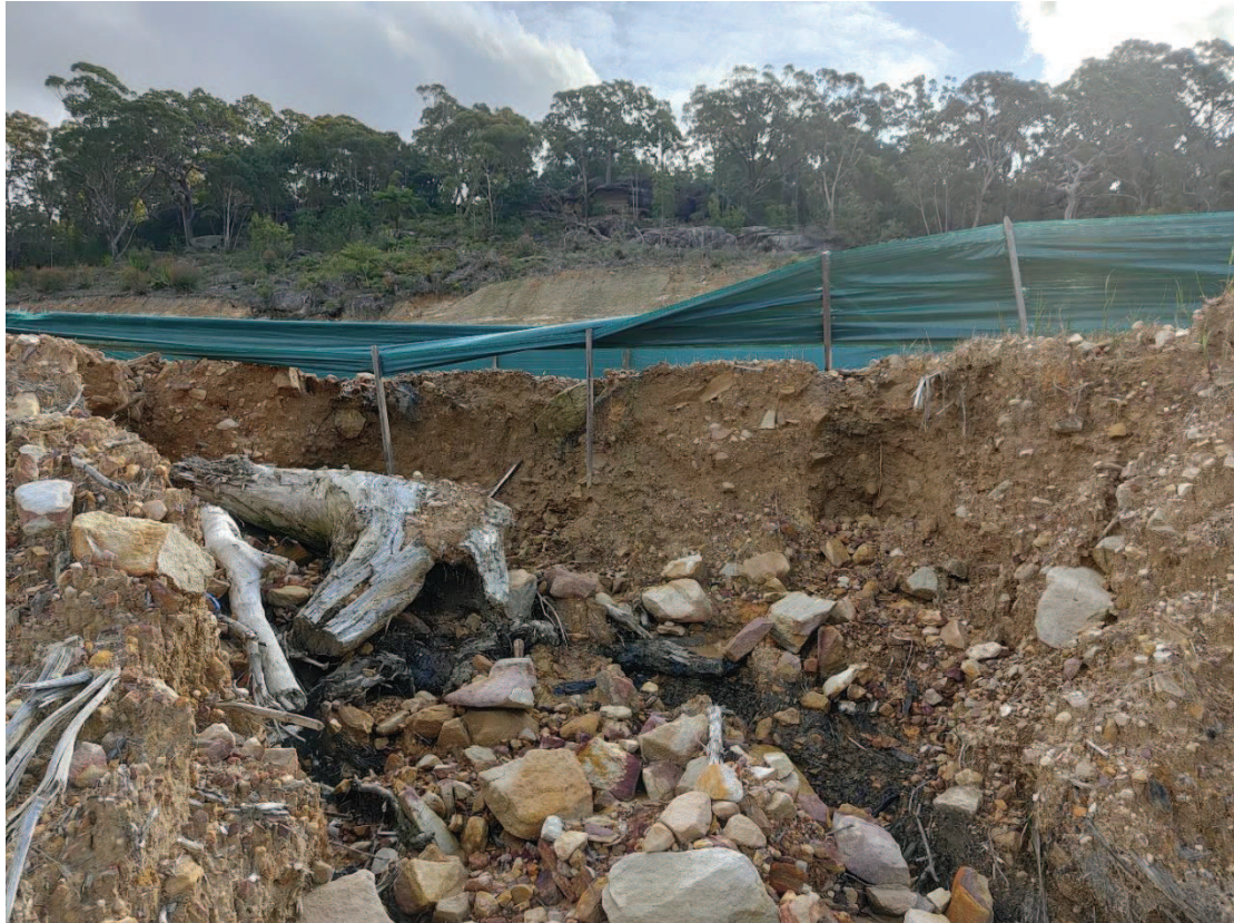
Photograph 4.1: Failed sediment control device on the Subject Land
